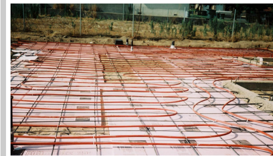
August 24, 2005 — Radiant heat tubes.
