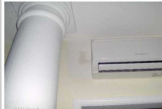
Jan 10, 2007 — HVAC installed
